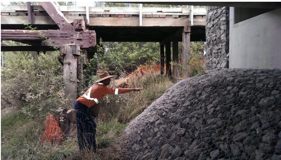
Photograph P13 - Approx. floodwater level from storm on 8 March 2014 at the western abutment of Gundaroo Bridge.
